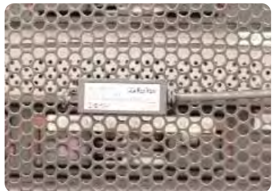
An example of a temperature sensor mounted at the cold air inlet of a server rack. Sensor is connected to an intelligent PDU (not shown).
